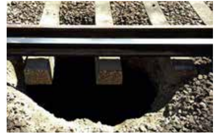
Sinkhole under railway tracks
